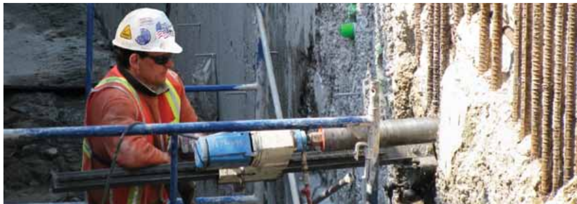
J. P. Hogan cored over a thousand picking holes on the slurry wall.
