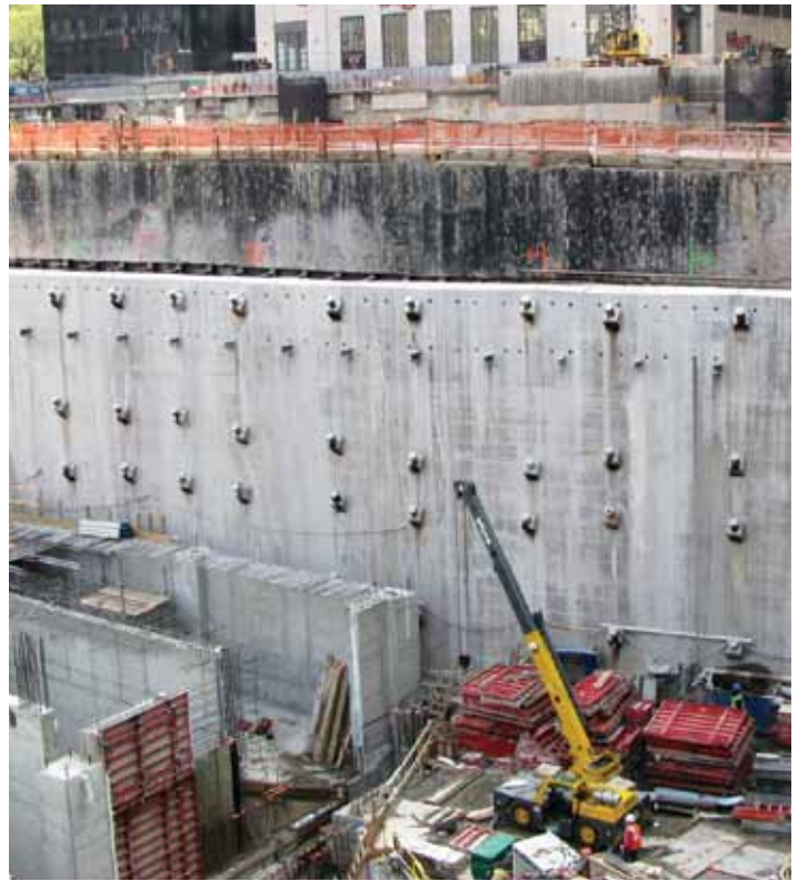
Demolition of the slurry wall will make way for the new construction.
