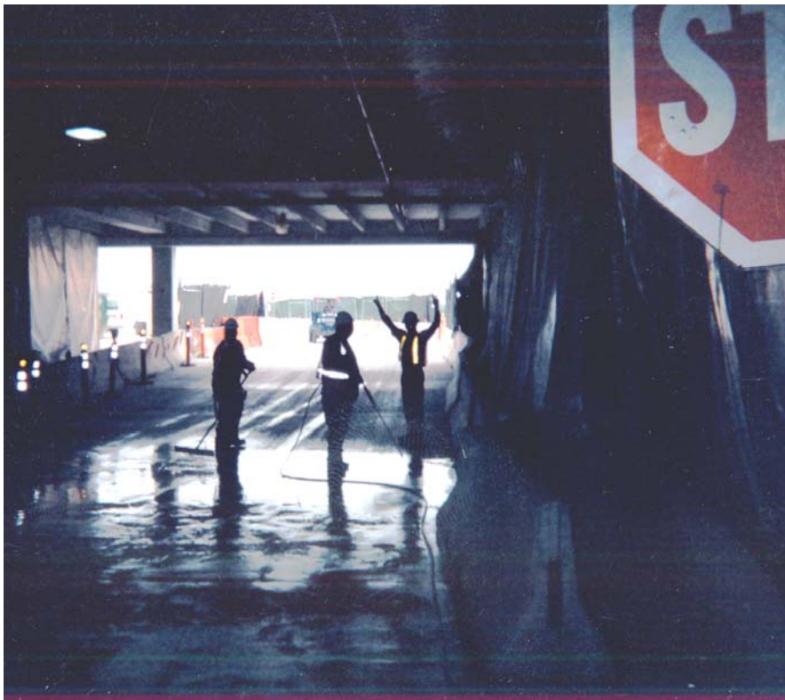
Crews were careful to secure the work area to protect airport personnel using the infill.
